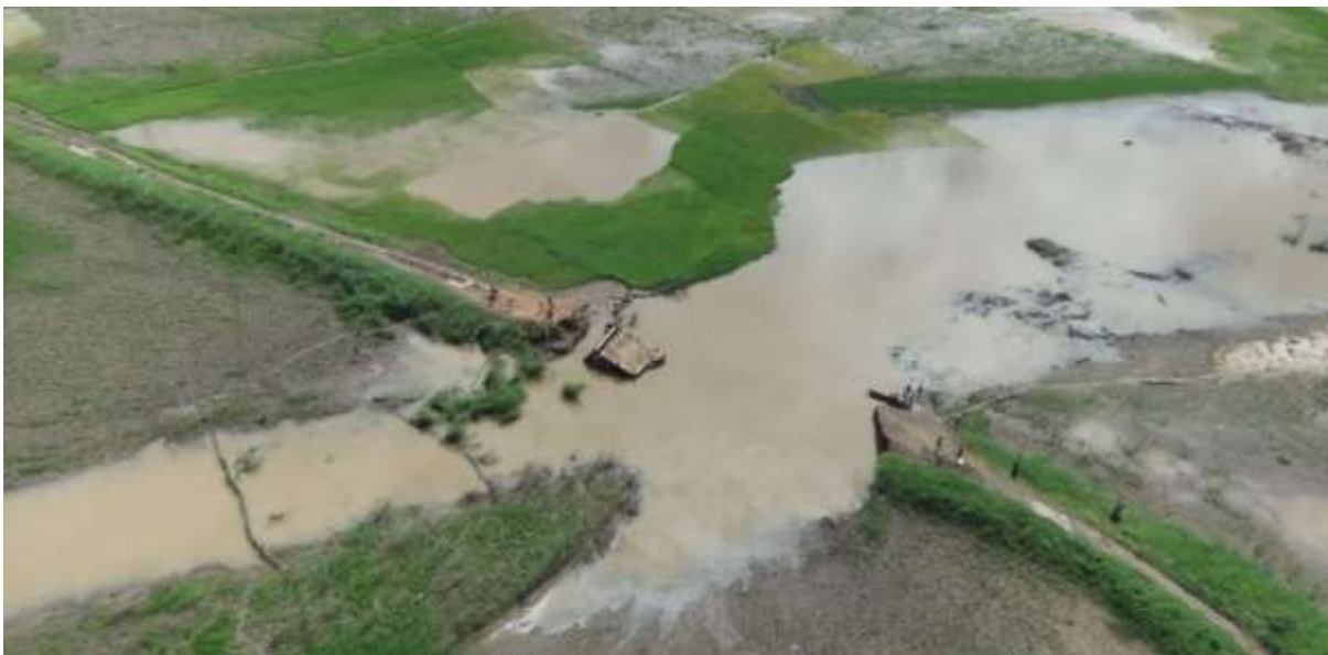
Figure 13 – Collapsed Bridge and Breach at Naminane
