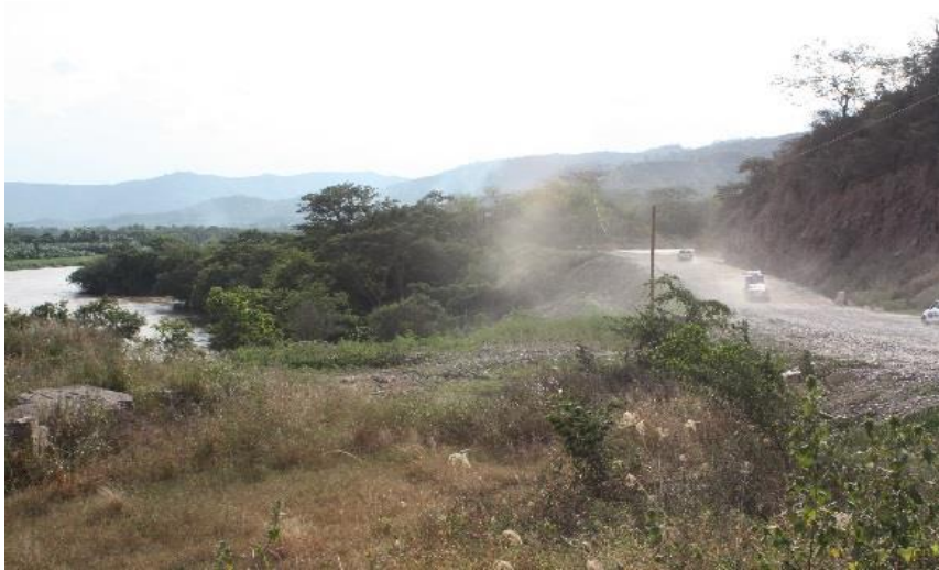
Picture 3-4 frequently inundated and damaged part of national road (Mayo/ Huallaga inflow)
