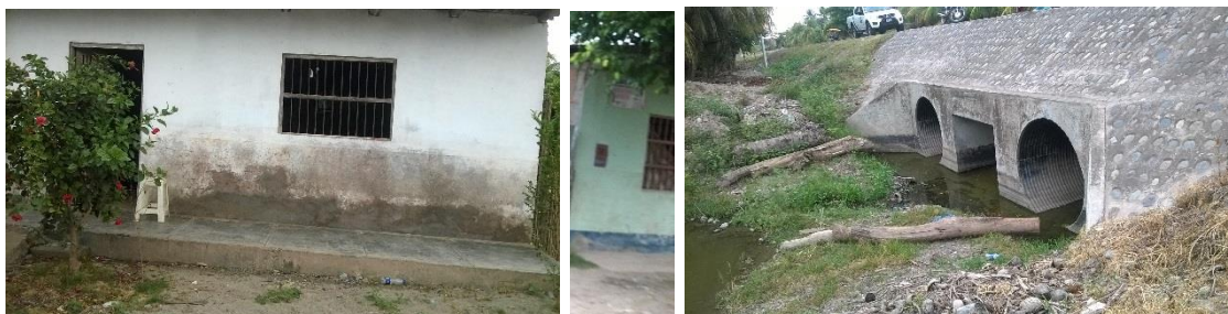
Picture 3-10 Bella Vista/La Libertad inundation lines visible at the houses and the culvert under the road
