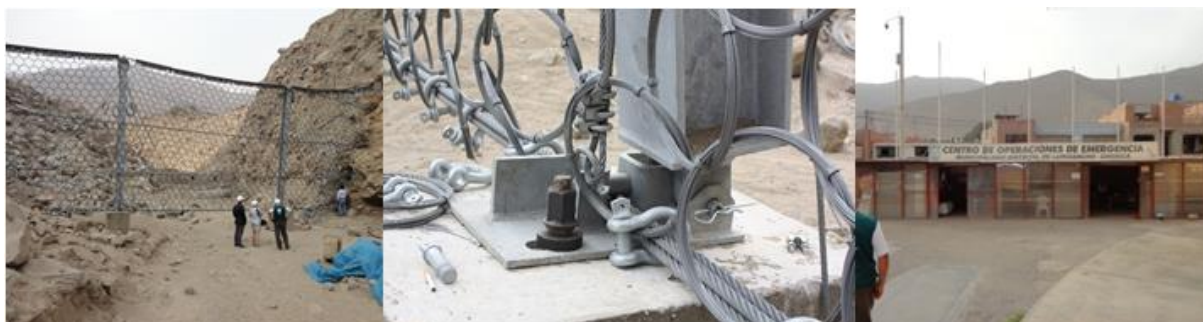
Picture 1-2 Impression of the installed mesh and Emergency operation centre in Chosica
