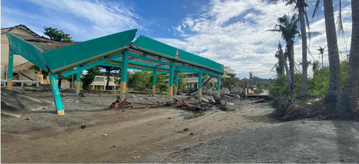
Figure 2-2: Damage in Antipolo National High School
