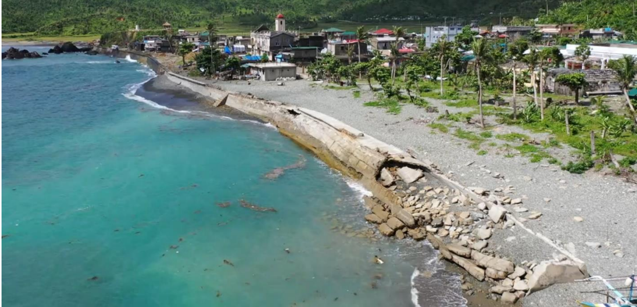
Figure 2-6: Seawall damage in JM Alberto
