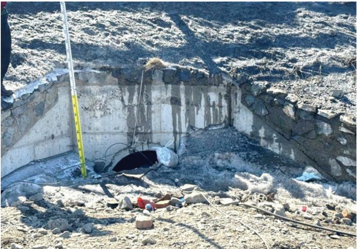
Figure 14a: Flood drainage facilities - A culvert trapped by sediment in "Gants Khudgiin Am" catchment (Source: Photo by IGG, MAS)
