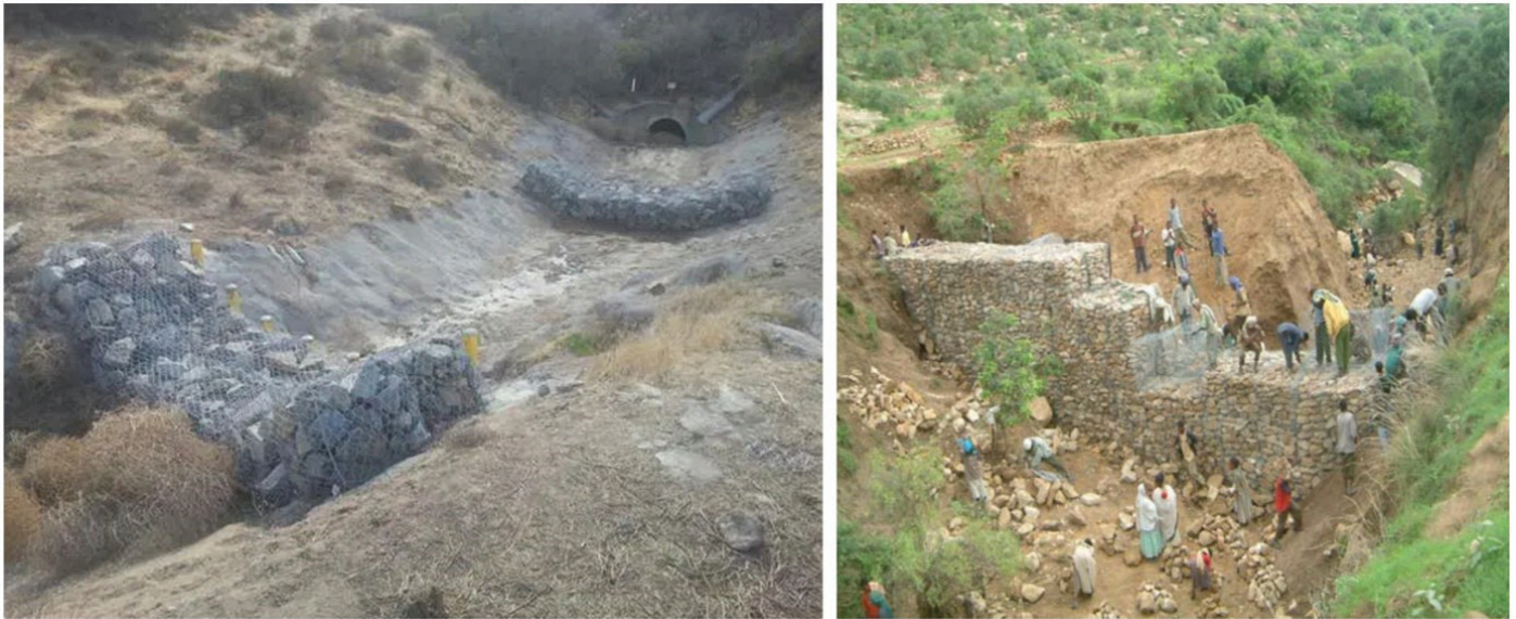
Figure 21: Examples of gabion gully plugs dams (from gabionsupply.com) (left) and Nile Basin Initiative (right).
