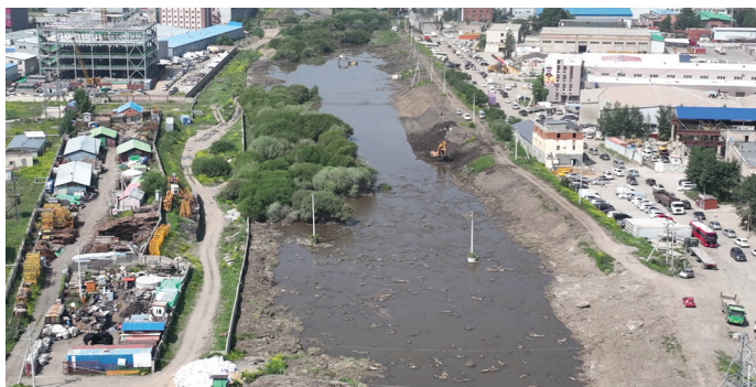
Figure 29: Bird-eye view on the Selbe River after excavation works in May-June 2024 (source: photo by GUBB).
