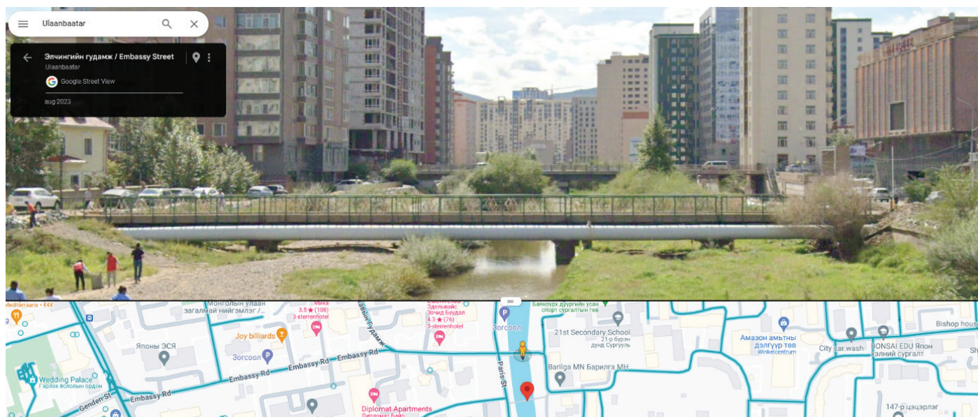
Figure 32: Photo of the footbridge south of Embassy street, demonstrating insufficient under bridge clearance (Google Maps Streetview August 2023). The top of the bridge is equal to the bank height. The bottom of the bridge deck and the heating pipes are all lower than the banks, largely obstructing the flow.
