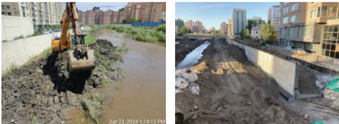
Figure 11: (left) construction works to the flood wall are ongoing in September 2024 (location left bank upstream of S-Outlet), (right) channel excavation works have enlarged the flow capacity of the channel downstream of S-Outlet. (Source: Photo by DRRS team)
