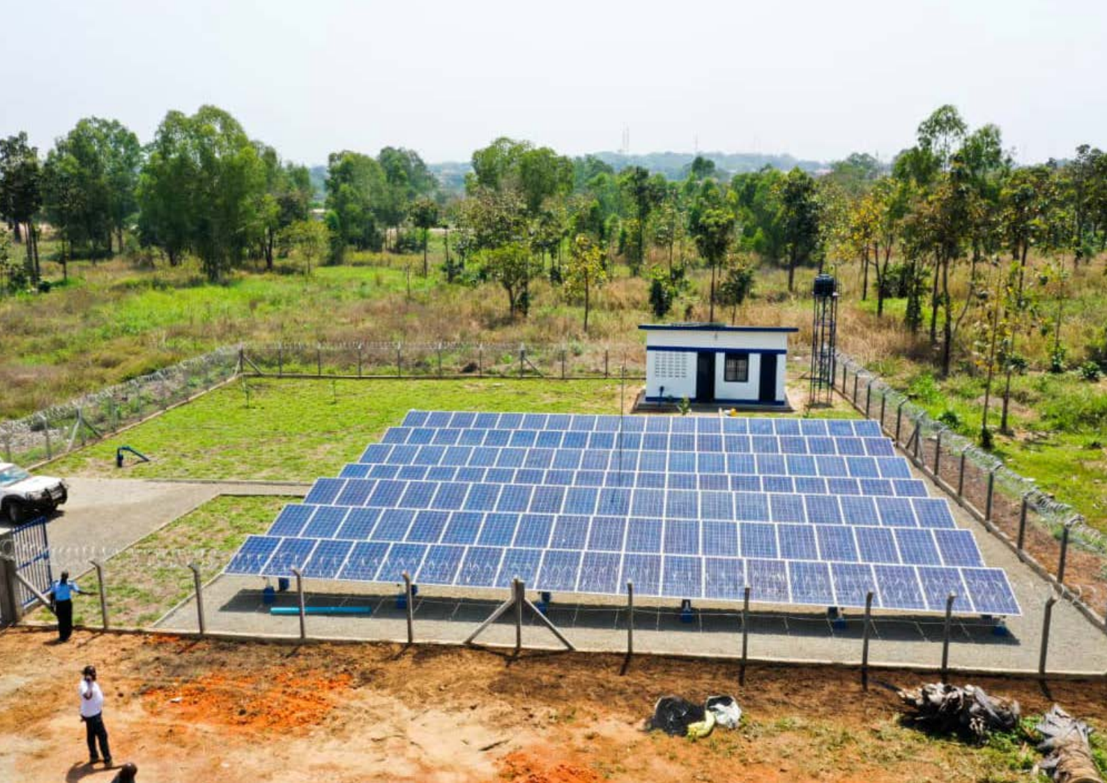
Renewable (solar) energy facility in Kitgum, Uganda, a more reliable power supply for the local water schemes.
