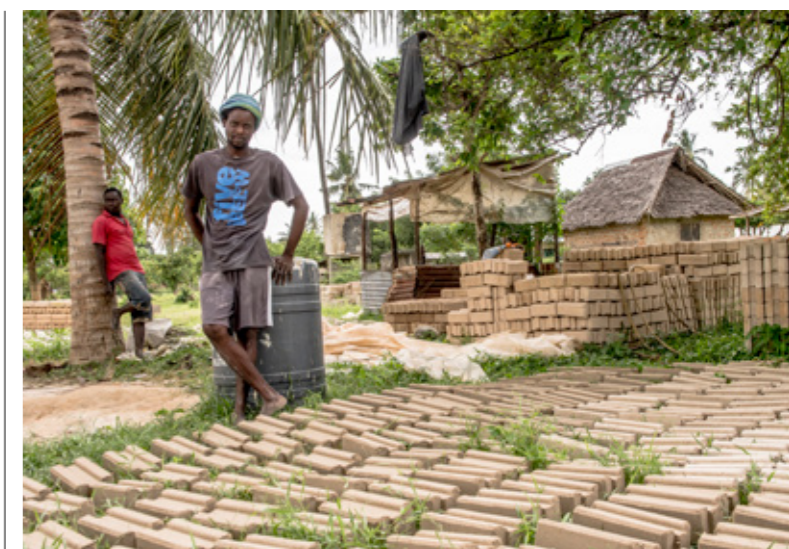
Roger Kalama Nguwa produces the special interlocking bricks used for the toilets
