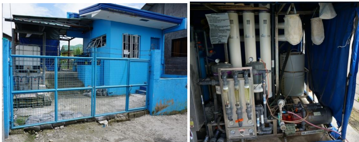
Figure 4.5: PS San Jose Gumi and mobile RO arsenic removal plant at PS San Jose Gumi
