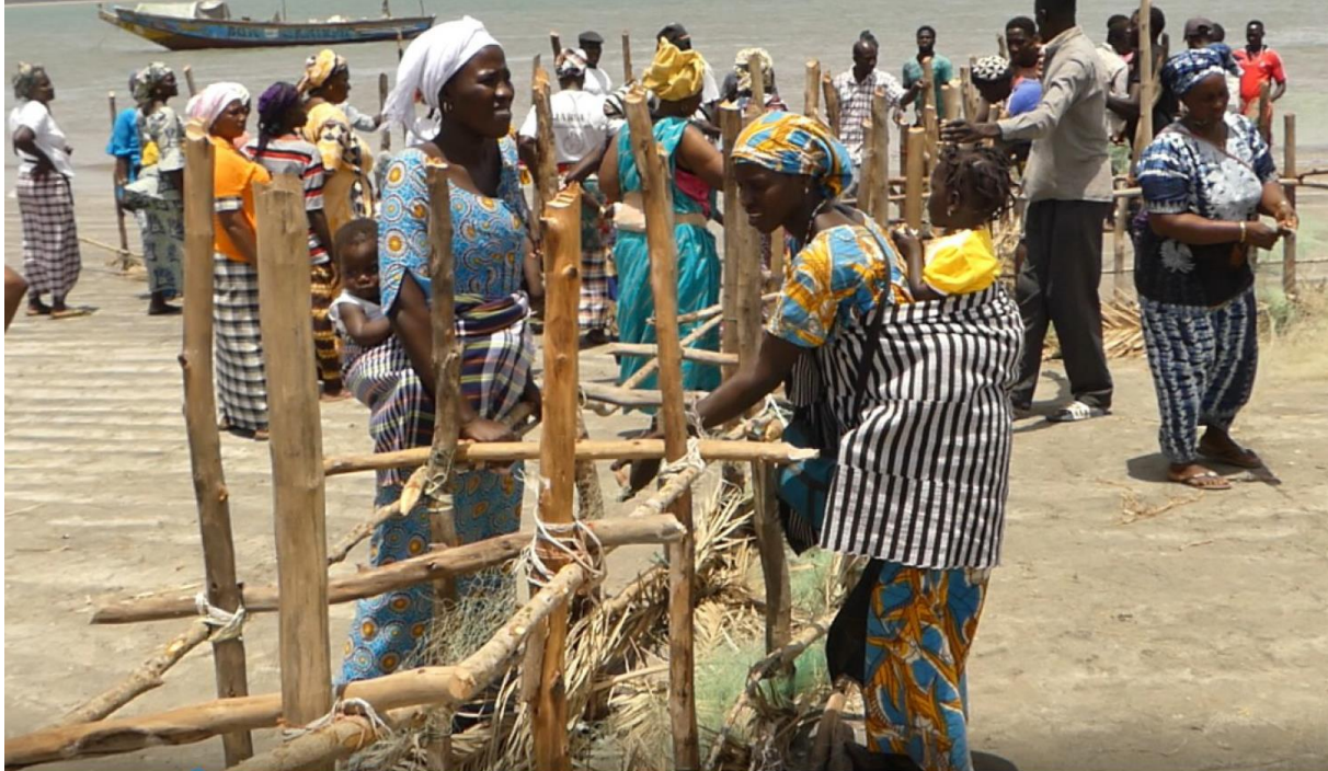
Figure 8 – Building the wooden groynes in Senegal was a community effort with 100 men, women and children from the village of Diogu  involved (photo: Patrick Chevalier). The day was concluded with festivities and a speech from the mayor.
